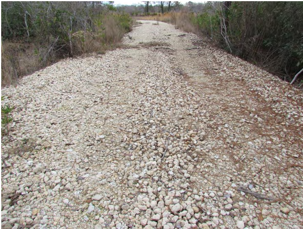
Photo 10. Low-water crossing and culvert (not visible in photo) that allow discharge from non-forested wetland. Photo point 3 facing east. 2/13/12. RTN
