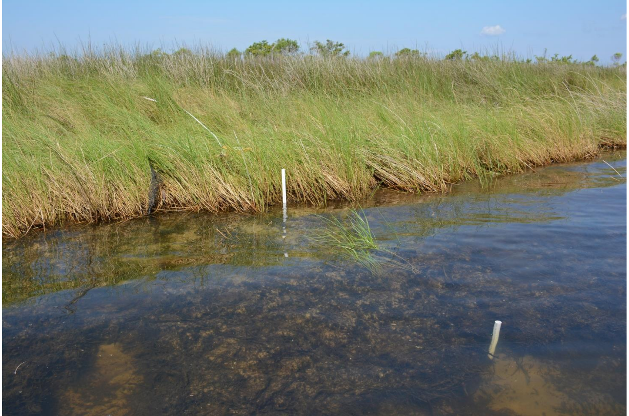
Figure 20. Undercutting of Salt Marsh (6/12/2019)
