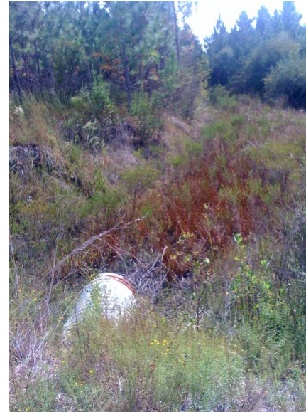
2. Existing culvert through pine plantation in western portion of the restoration area
