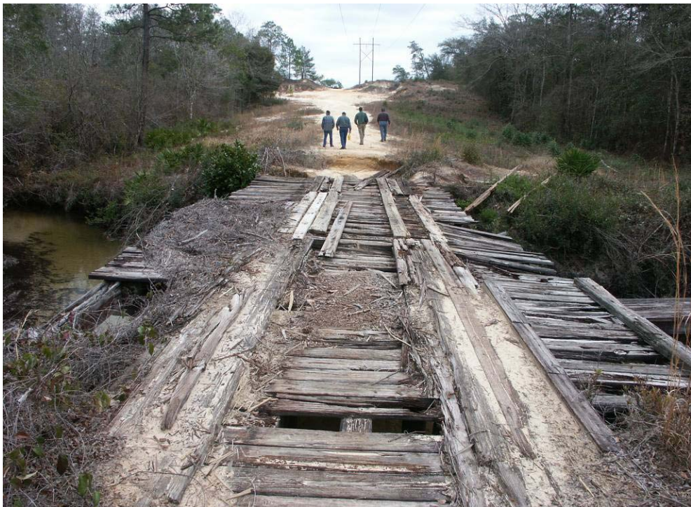
Failed bridge over Wolf Creek
