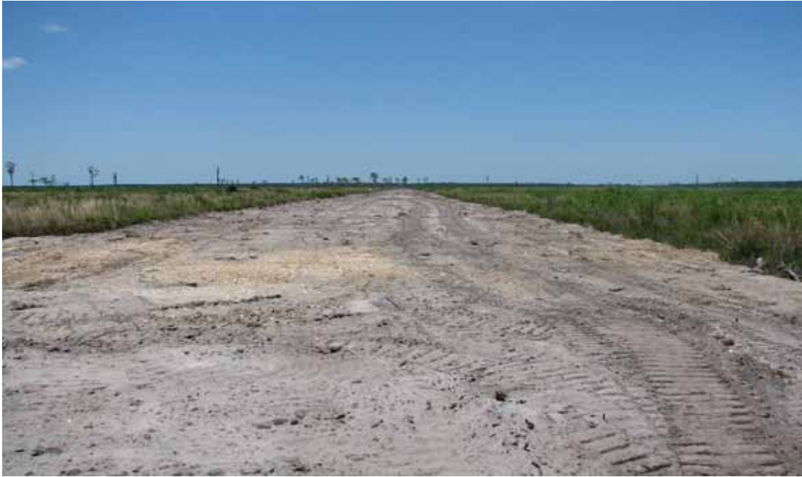
Figure 5. Road removal site #2 (easternmost road) after roadbed was pushed into adjacent ditches and contoured to existing adjacent natural grade.
