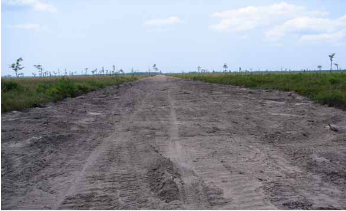
Figure 3. Road removal site #1 (westernmost road) after roadbed material was pushed into adjacent ditches and contoured to existing adjacent natural grade.
