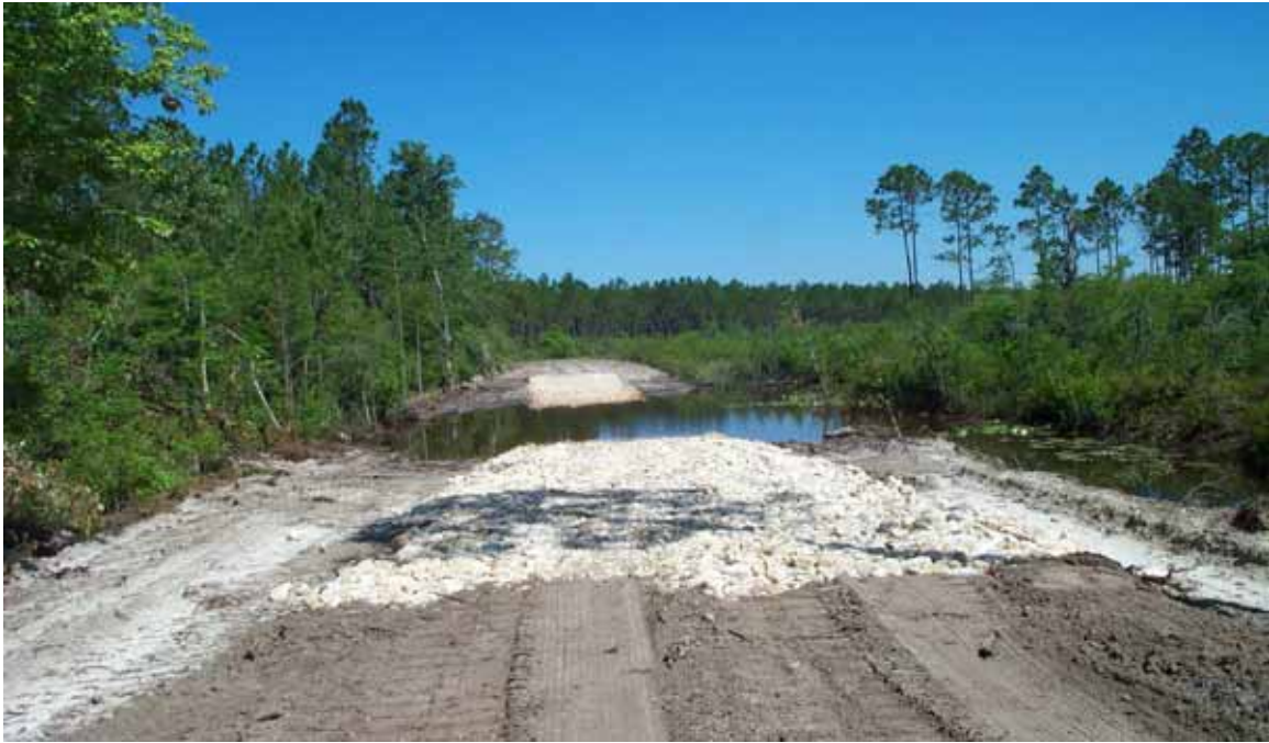
Figure 7. Hardened low-water crossing at site #4 after completion of construction. Water is flowing from right to left across the structure after a recent rain.
