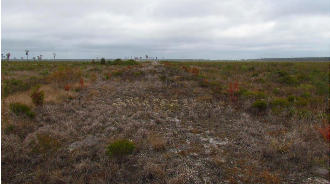
Photo 1. Road removal; roadway edges lined with planted cypress showing fall color. Photo Point 1, looking north. 11/16/2011
