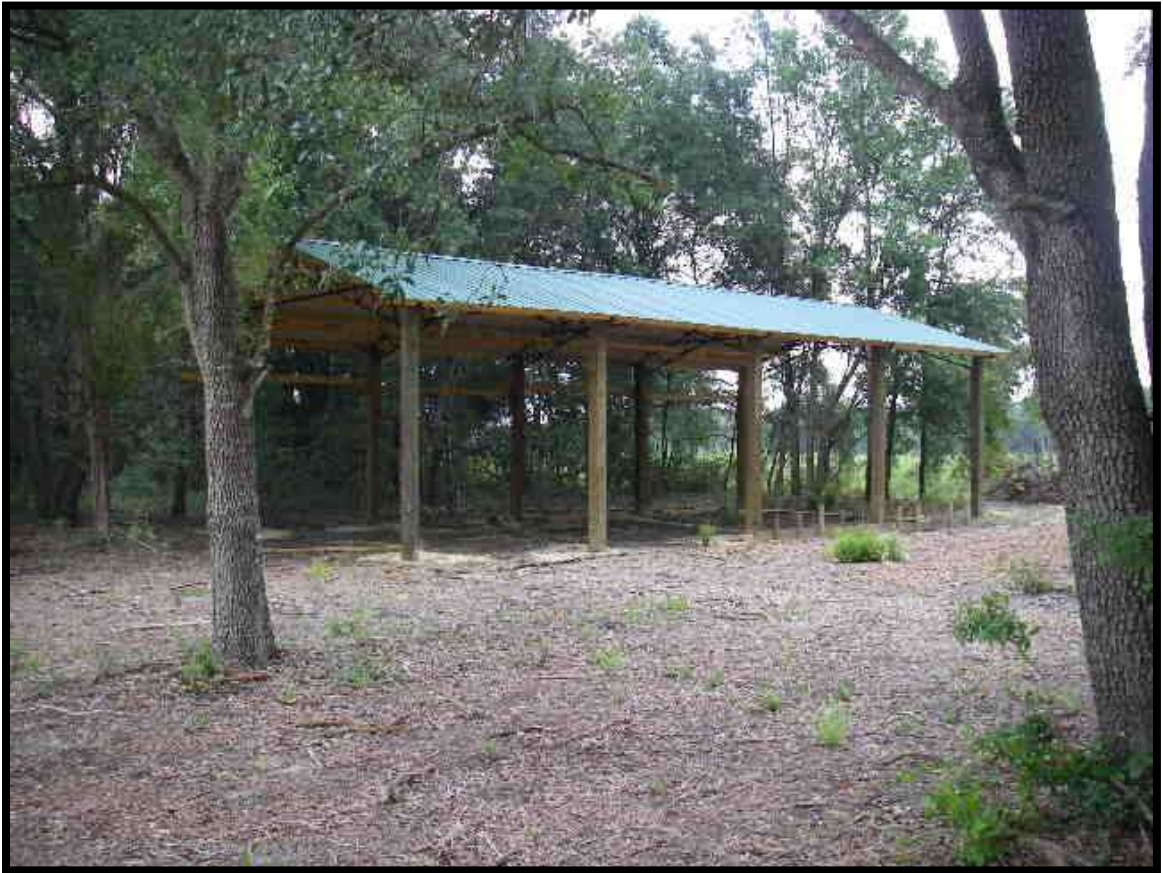
Figure 3. The NFWFMD began construction during July 2010 on an equipment storage shed that will also provide two open bays for storage of boats and ATVs for the area.
