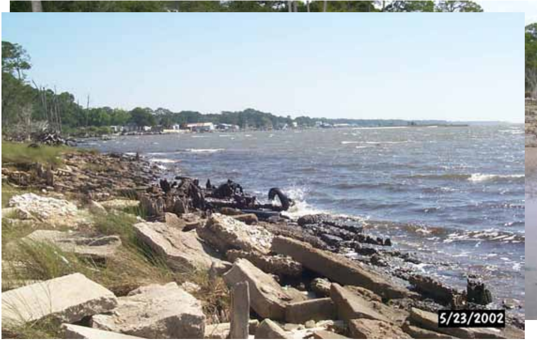
Figure 4. Preconstruction view of concrete construction material previously placed on site to control erosion of shoreline.
