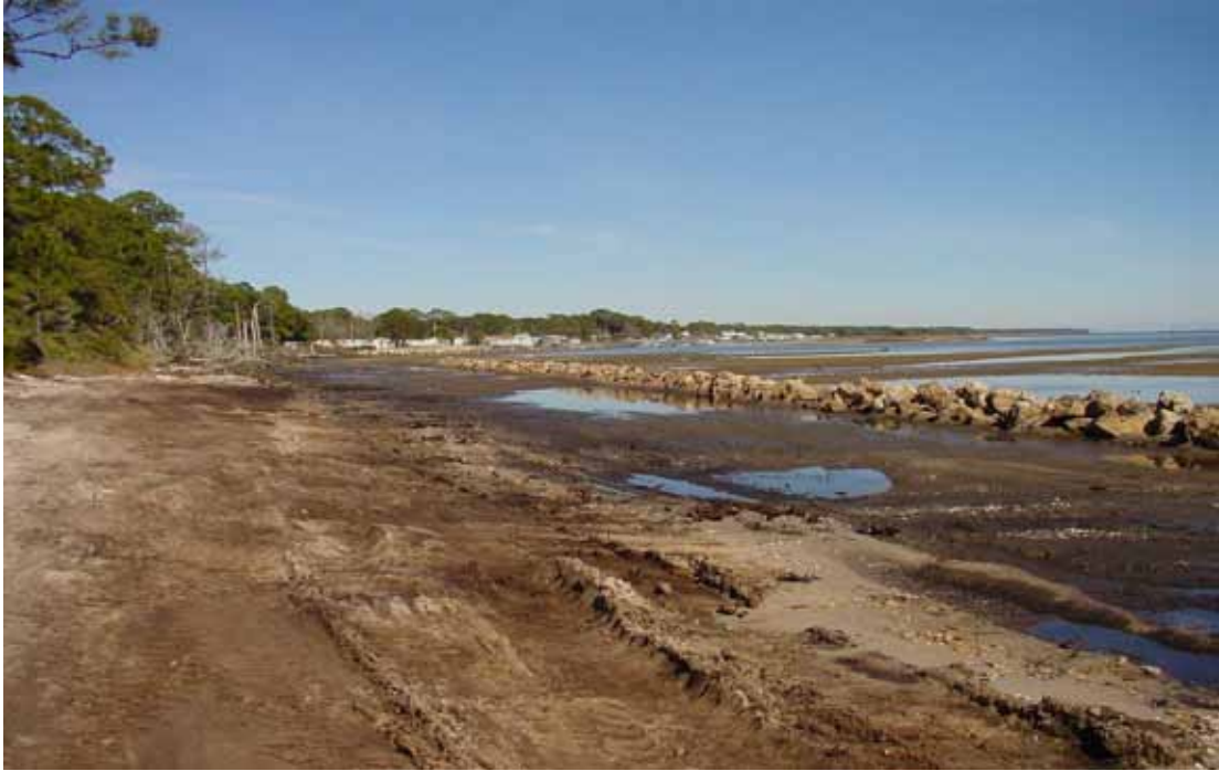
Figure 10. Construction of breakwater complete along with rubble removed and shoreline sloped to match adjacent beach profile.
