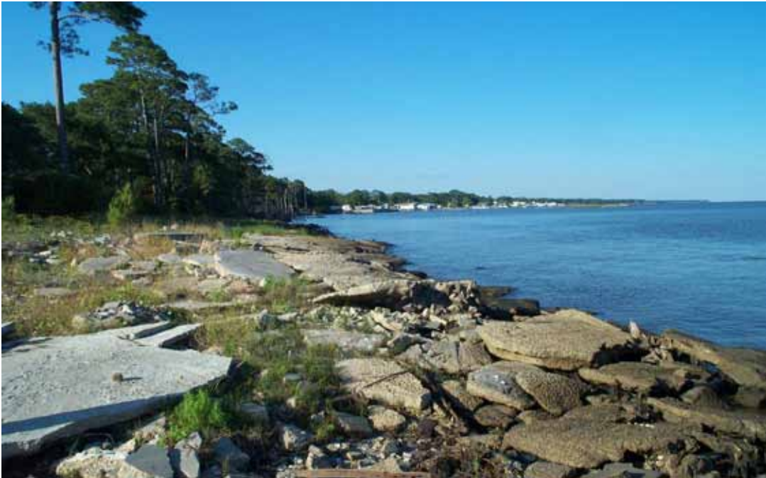
Figure 5. Preconstruction view of concrete construction material previously placed on site to control erosion of shoreline.
