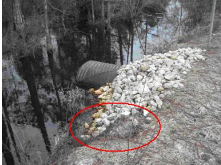
25. Whiskey George Tract. C1. Circled area highlights minor bank erosion.
