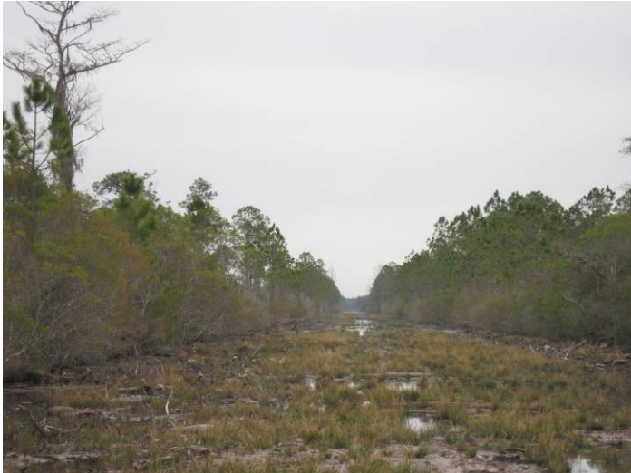
1. Sumatra Tract. Segment 5. Under-excavated road segment
