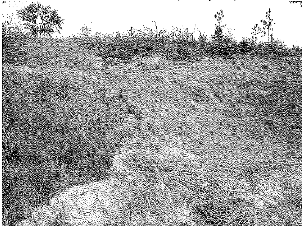
Cat Pond Erosion Restoration Sites #1 and #2 (February 2007)
