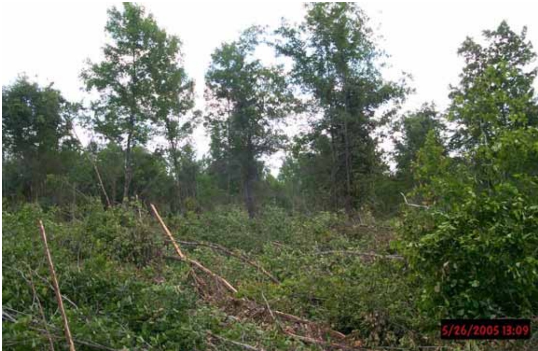
Figure 4. Appearance of site after initial walkdown of vegetation. Most trees and shrubs less than 6-8 inches in diameter have been pushed over and are awaiting roller chopping and fire.
