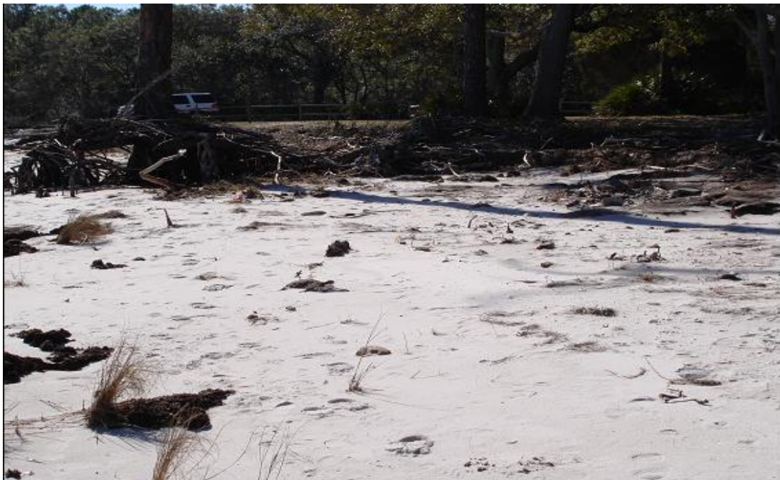
Figure 11. Erosion and scour in upland buffer zone in middle of site. Annual monitoring photo shows an additional loss of 15-20 feet of upland that occurred during the 2008 storm season.
