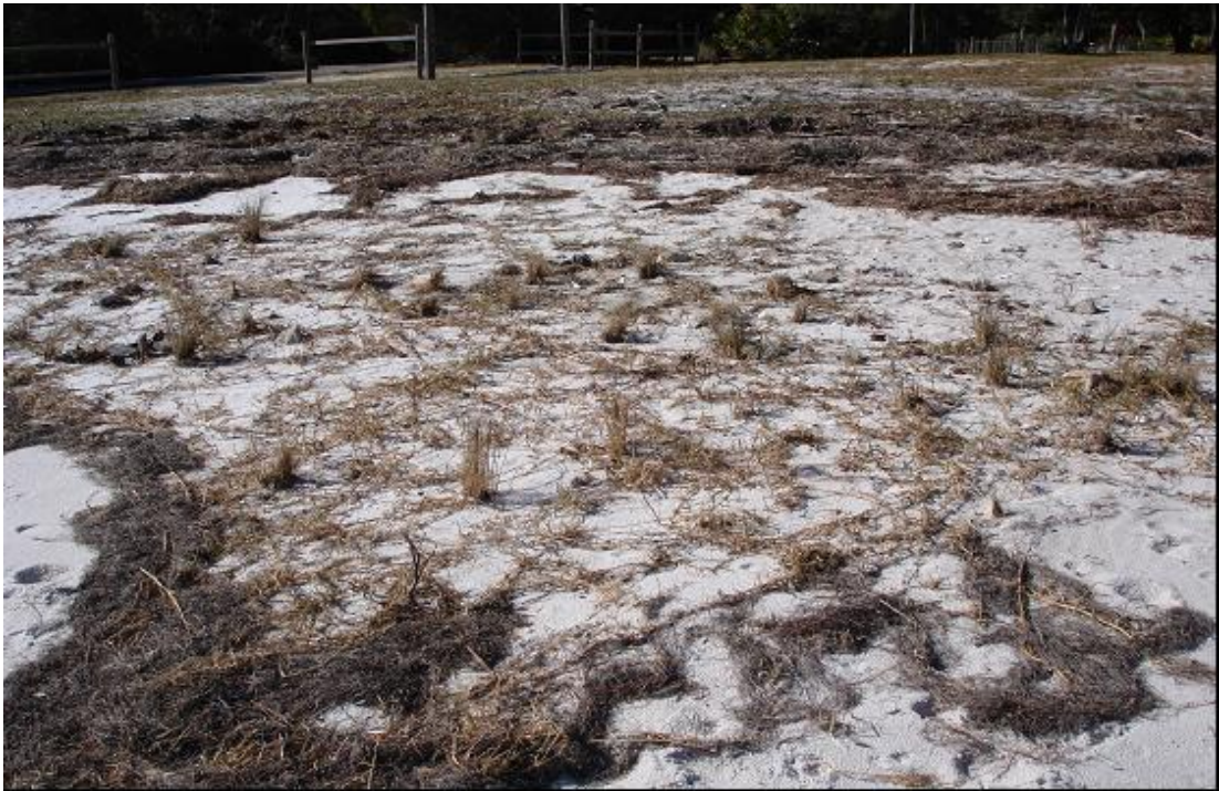
Figure 13. Significant erosion and scour of upland resulting from high storm surge. Surviving saltmarsh cordgrass and sea purslane in southern portion of upland buffer (noted in annual monitoring 2008).
