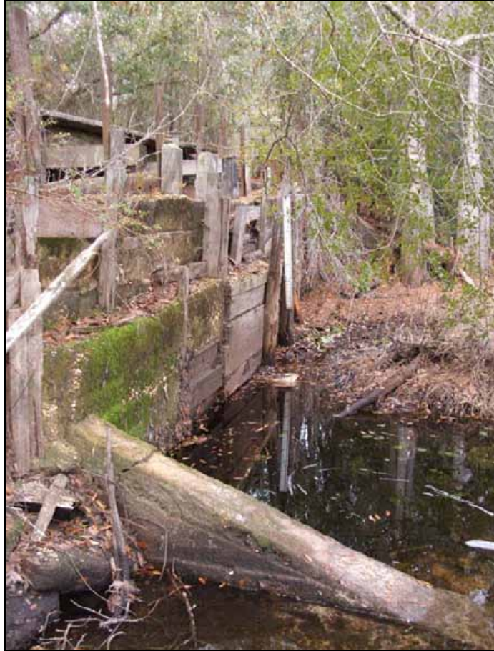
Figure 57. Photograph of the north side of 8WS469, view to northwest. Note the concrete buttress and foundation that extends below the majority of the structure, including the horizontal planks shown here beyond the concrete buttress and dam wall segment.
