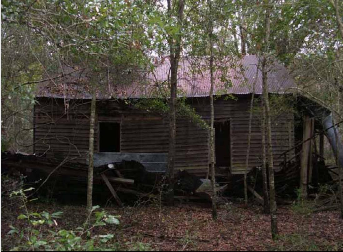
Figure 65. Photograph of 8WS471; view to the east looking at west side of the structure.
