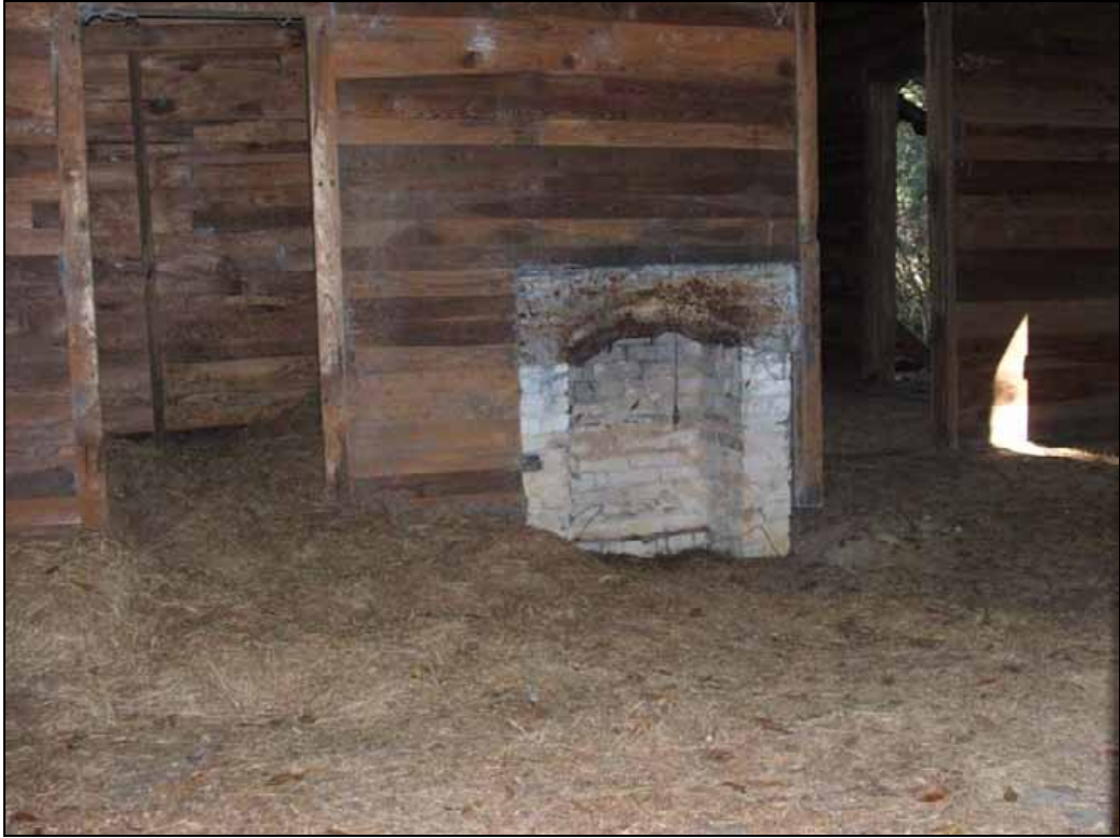
Figure 66. Photograph of 8WS471; view of the interior of the structure from a window near the southwest corner.
