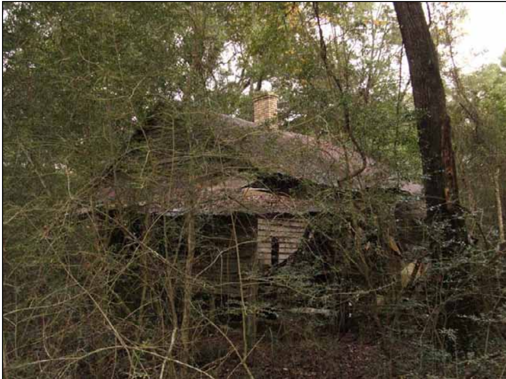
Figure 64. Photograph of 8WS471; view to the northwest looking at the southeast corner of the structure and small addition or detached kitchen.
