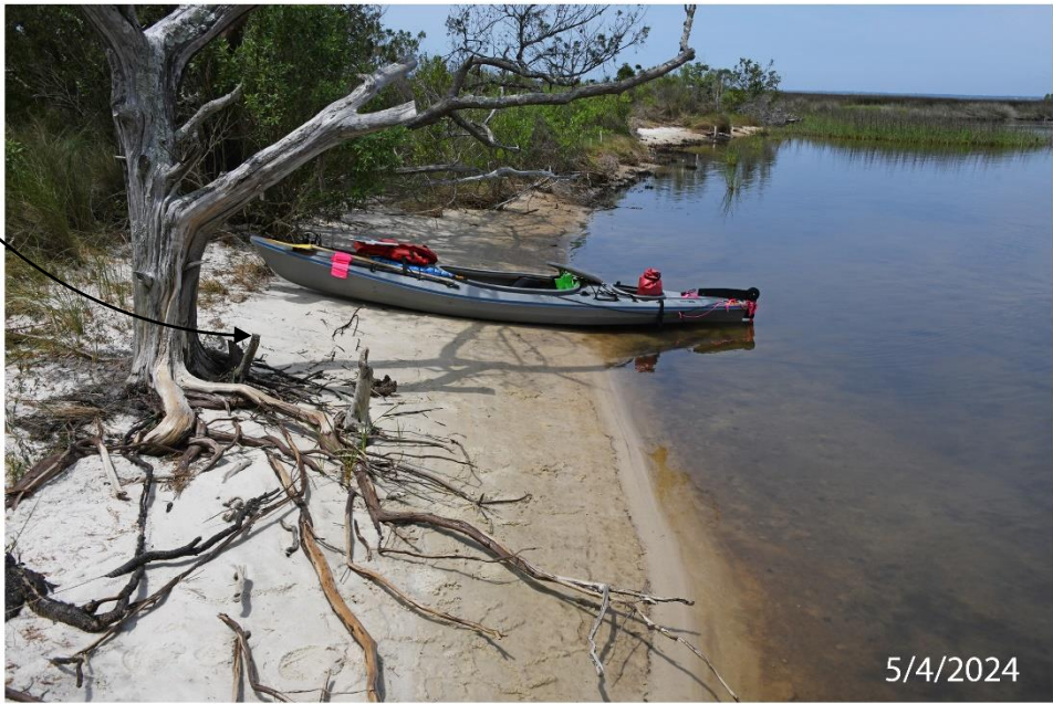
Figure 36. Washout of Planted Vegetation Not Protected by Breakwaters
